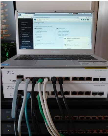
Figure 105 Cluster OPNSense & Switch
